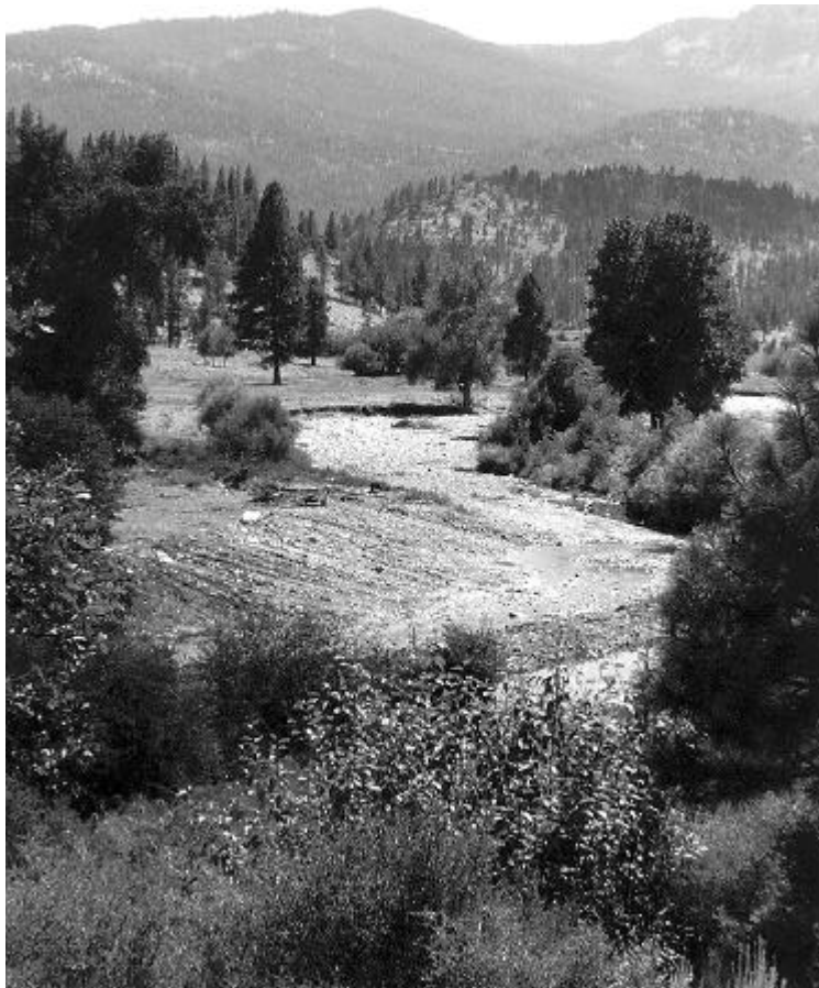
Figure A5-28. East Fork Scott River after excavation with heavy equipment under emergency flood relief. July 1997.
