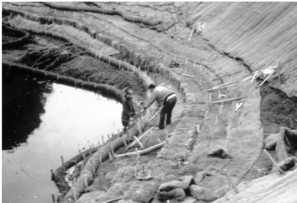
Figure 3. Installation of coconut fiber rolls and carpets secured with "two-by-four" stakes and polypropylene cord (October 1993).
