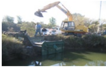
McBain and Trush recently completed construction of a 'fish friendly' tide gate allowing fish passage into Rocky Gulch.
