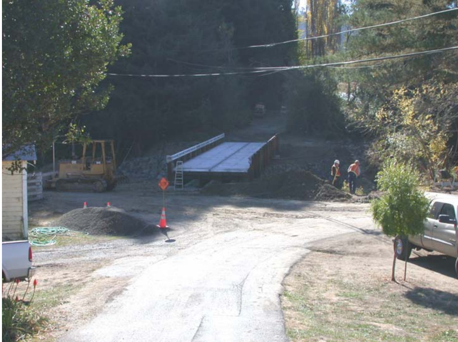
View looking from right bank to left bank after two-part bridge was set in place on concrete footings.
