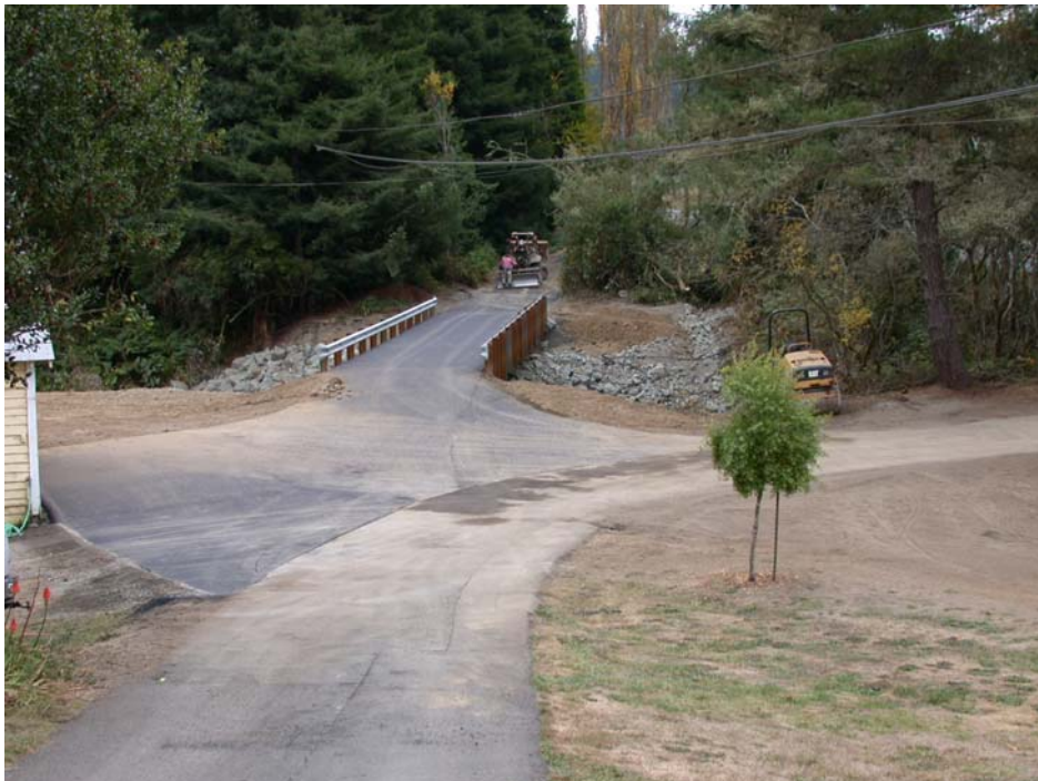
Same view as above after the banks have been rocked and mulched and the bridge has been paved.
