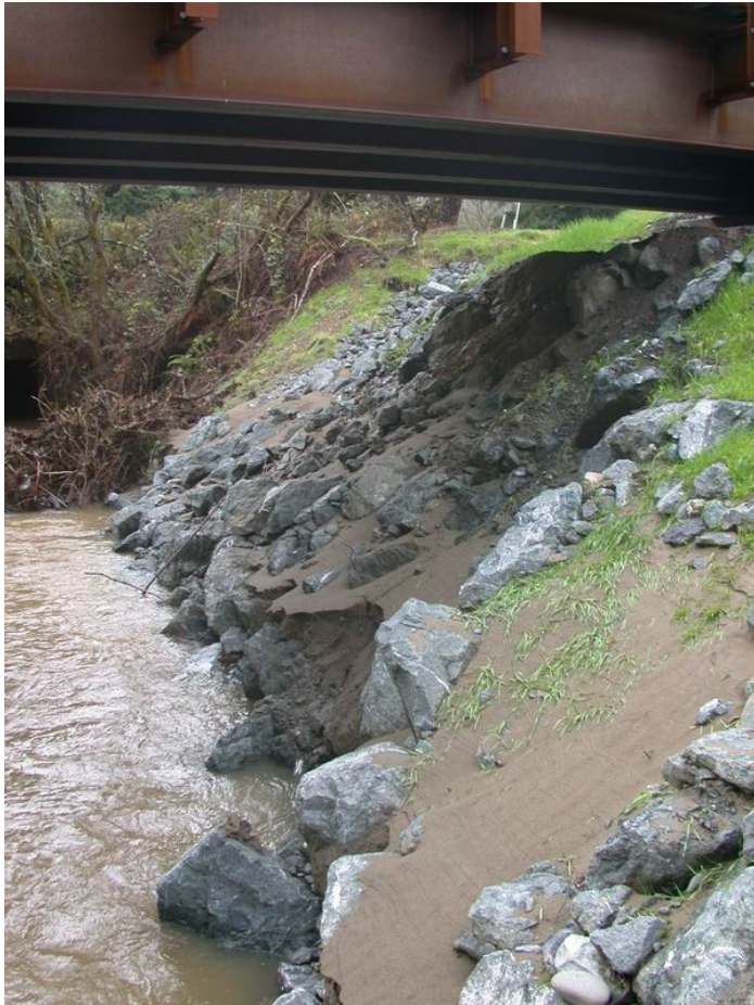
Picture looking downstream after project completion showing right bank fine sediment deposition.
