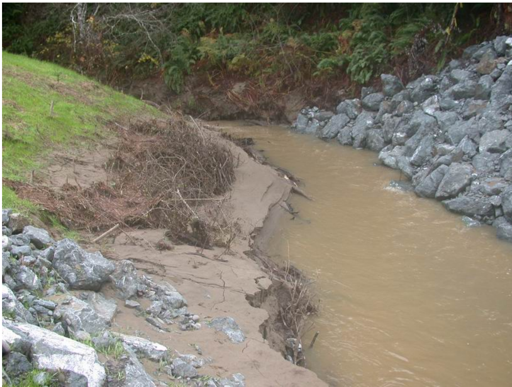
Looking 100ft downstream of bridge at sediment deposition on the willow mattress.
